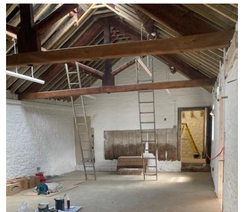
Above: Cart Horse Stables taking shape preserving what remains of the old kicking boards.
